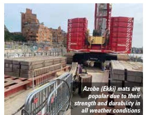
A crane operator in Waterford, Ireland had a lucky escape when his 50 tonne crawler crane overturned when the ground gave way
