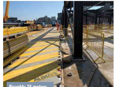
Roughly 75 metres long, the track was made up of 354 Alimats interlocking mats in three module sizes
